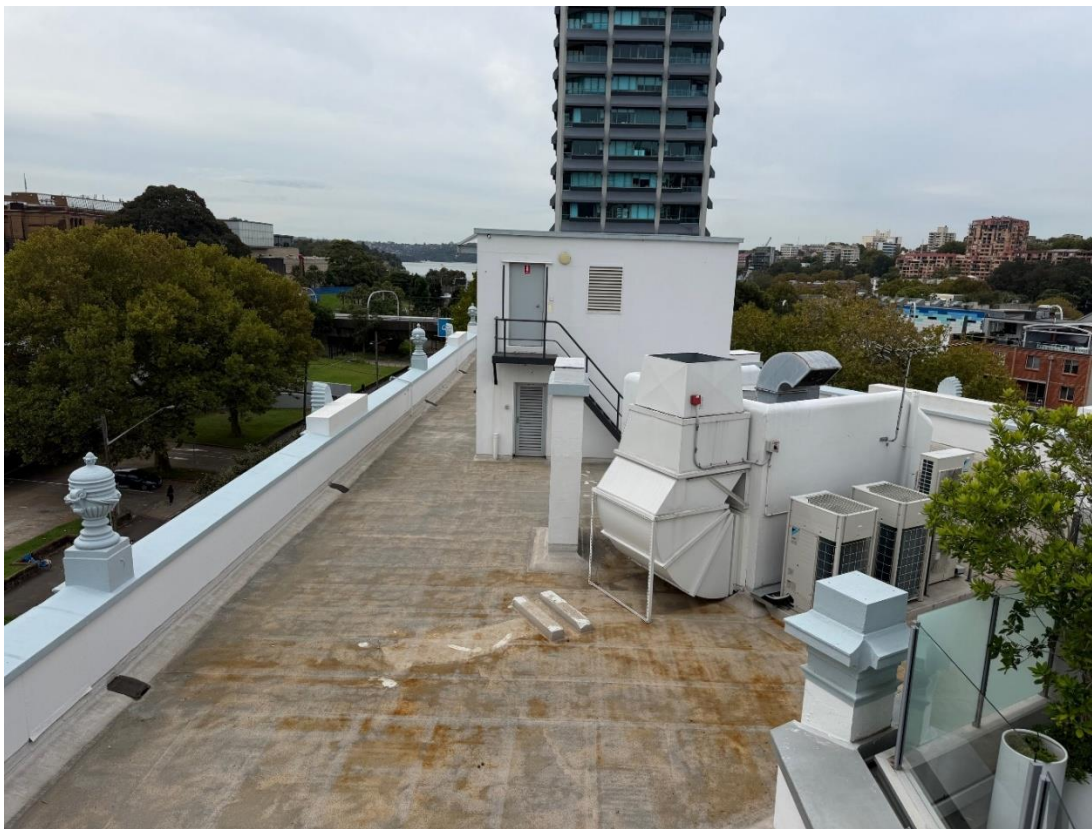
Figure 26: Balcony viewed facing north at Unit 51/62-68 Sir John Young Crescent
